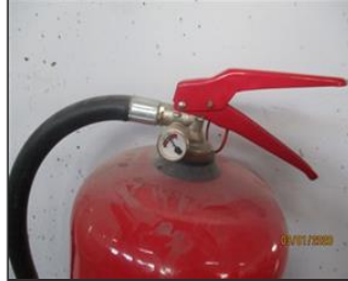
External photo(s) of the production unit(s) pressure of fire extinguisher.jpg
