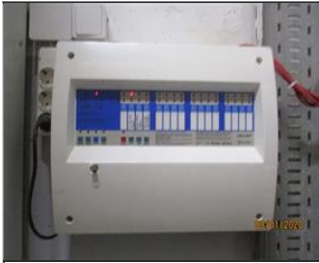
External photo(s) of the production unit(s) fire alarm control panel.jpg
