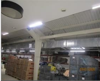
External photo(s) of the production unit(s) ventilation system.jpg
