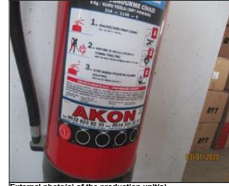
External photo(s) of the production unit(s) control date of fire extinguisher.jpg
