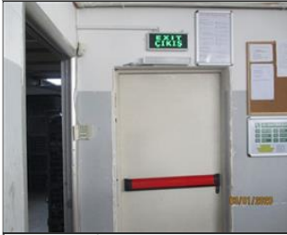
External photo(s) of the production unit(s) emergency exit door.jpg
