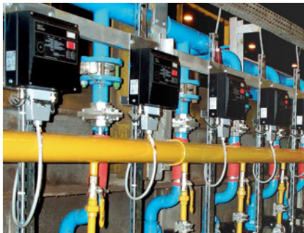
Hardening furnace with lots of industrial burners located side-by-side
