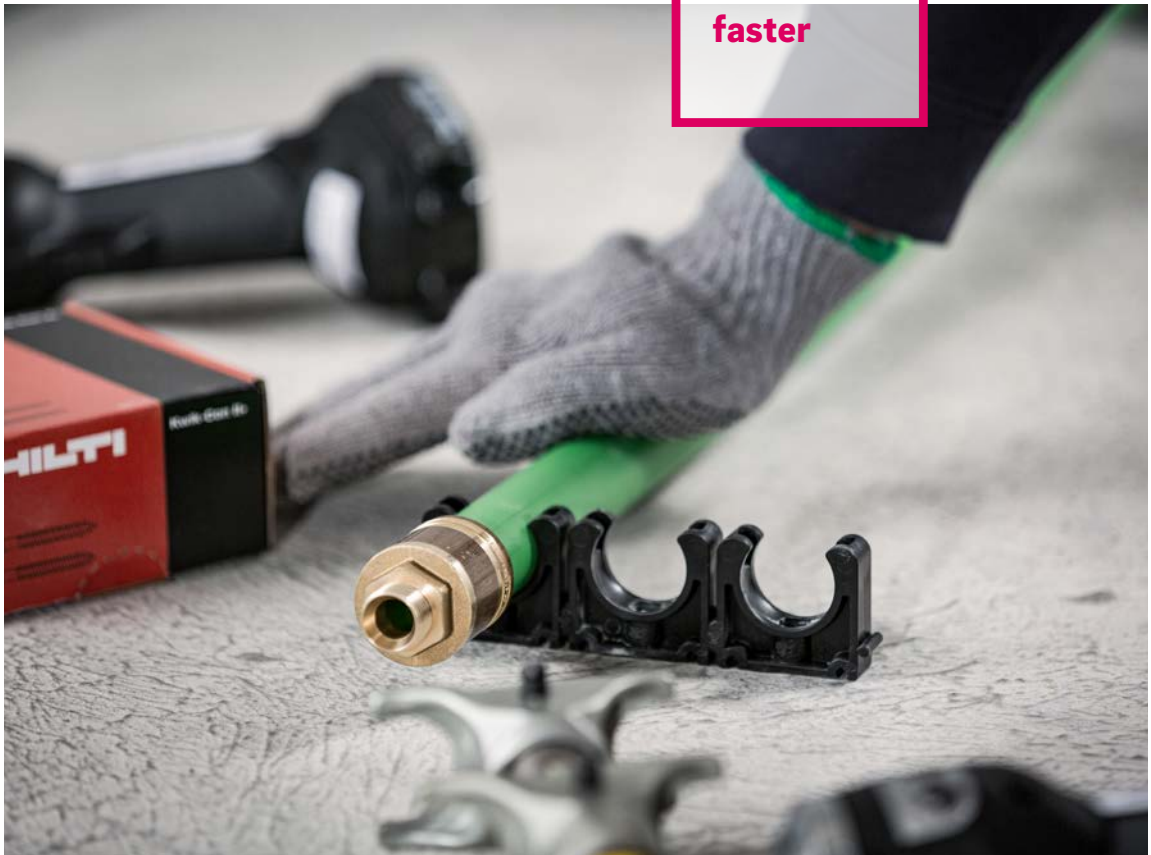
REHAU pipe clamp used for ground floor installation.
